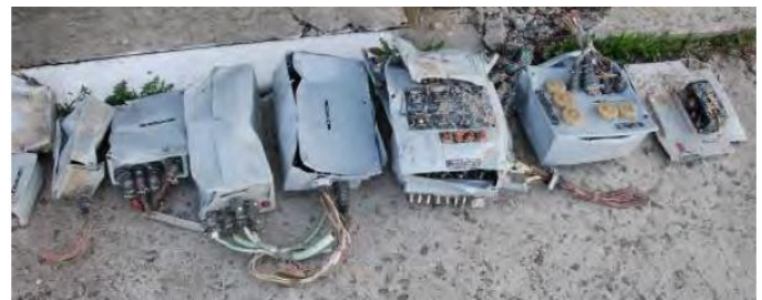
Fig. 13. Junction and control boxes of electrical installation. Photo taken at the site of wreckage storage [4].
